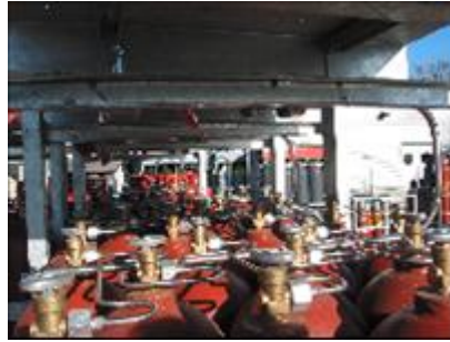
Fig 2 Pigtails used in a cylinder bundles installation
