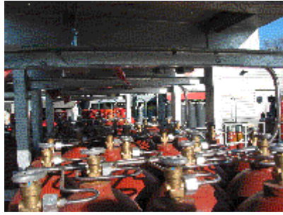
Figure 2 Pigtails used for an installation of bundles of cylinders
