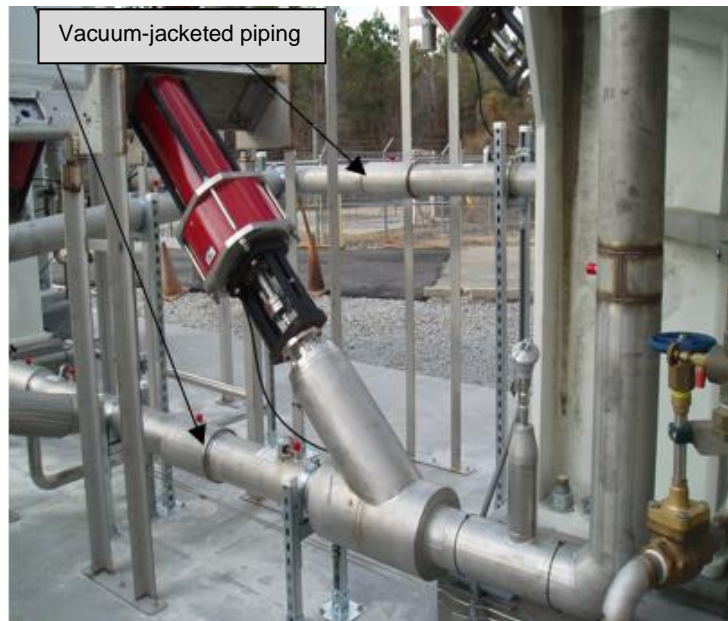
Figure 2 Example of a vacuum-jacketed piping run in service
