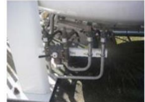
Typical tank relief valves
