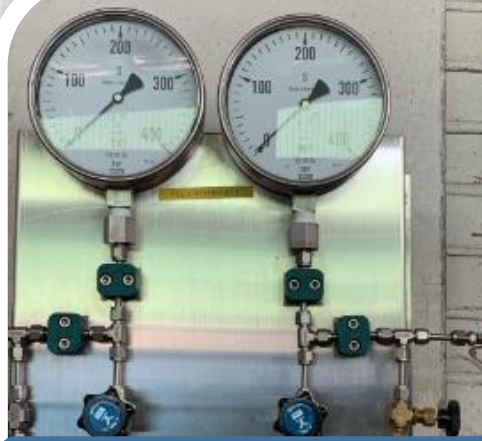
Fixed Monel Pressure Gauge Panel
