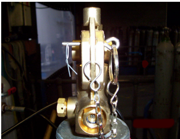
Figure 1—Cylinder valve with valve closed and locking device engaged
