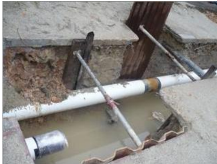
N2 pipeline cap and O2 pipeline
