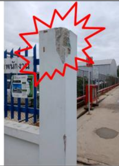
Damaged concrete gate post
