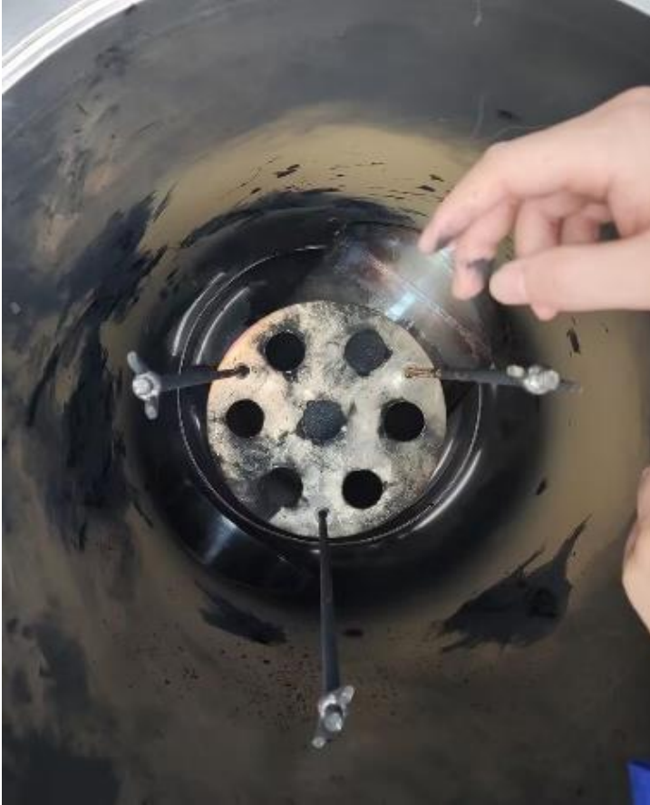
Internal picture of the filter after the fire
