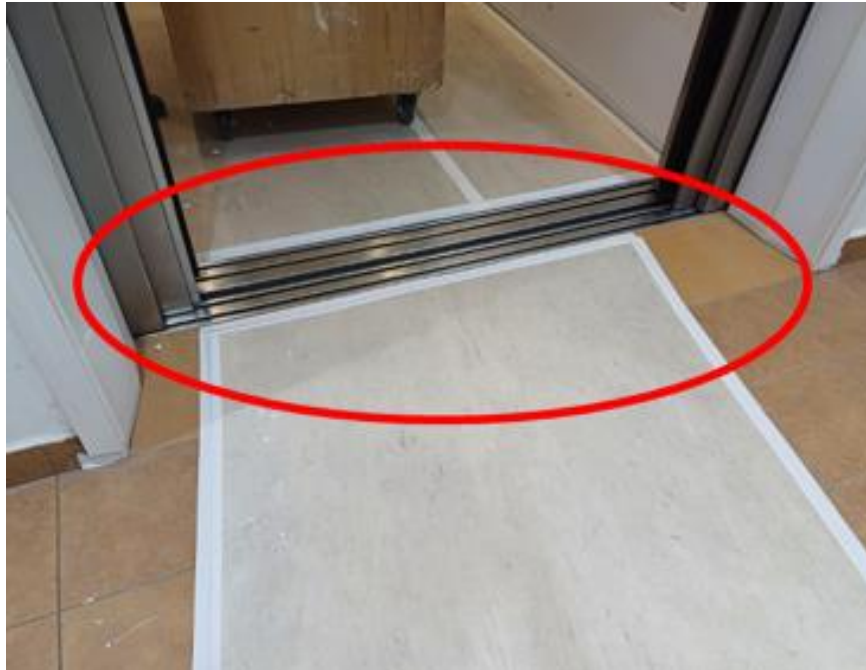
Uneven floor height between cargo lift and floor
