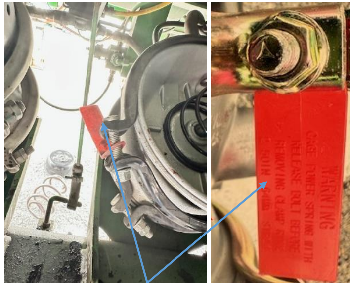
Warning label of stored energy in spring
