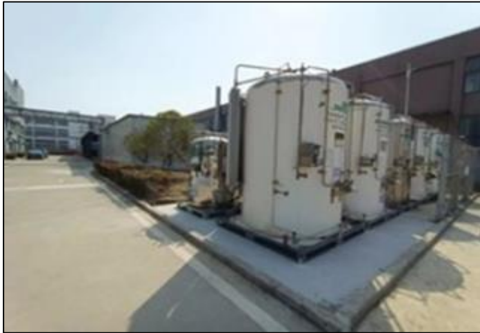
Some MB tanks interconnected together
